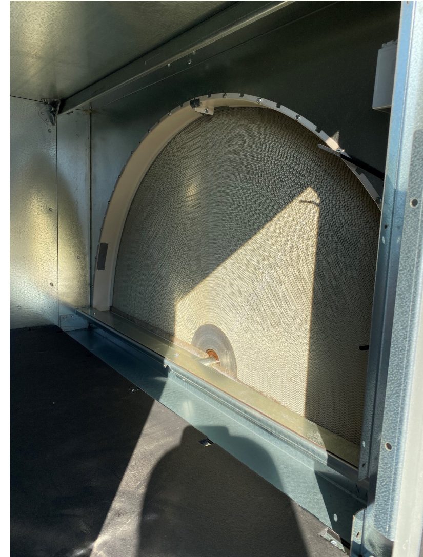
Return Air Side
