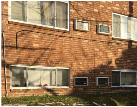
Existing Thru-wall Air-Conditioning
