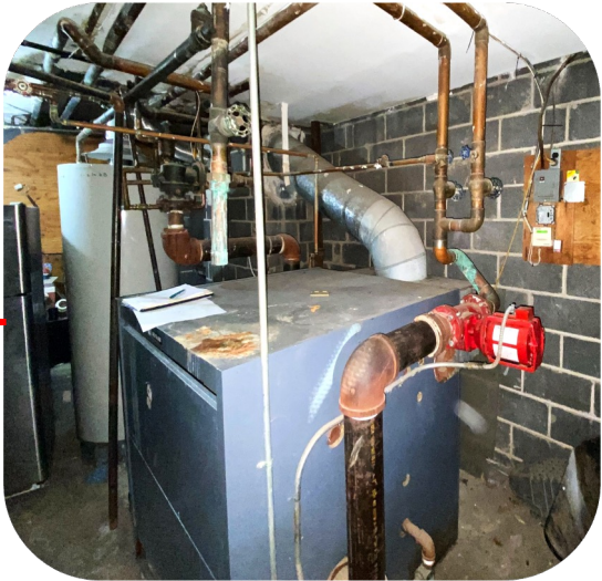
Existing boiler and gas HW heater
