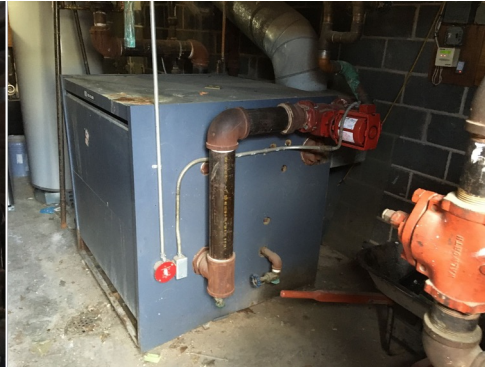
Existing Centralized Gas Boiler for Heating
