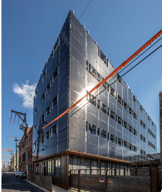
Front Flats, 174 kW array, Phila, Onion Flats
