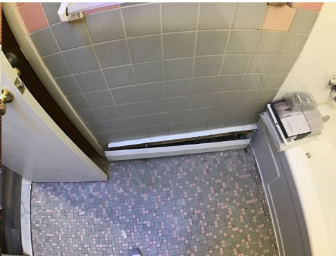
Existing Hydronic Baseboard Heating
