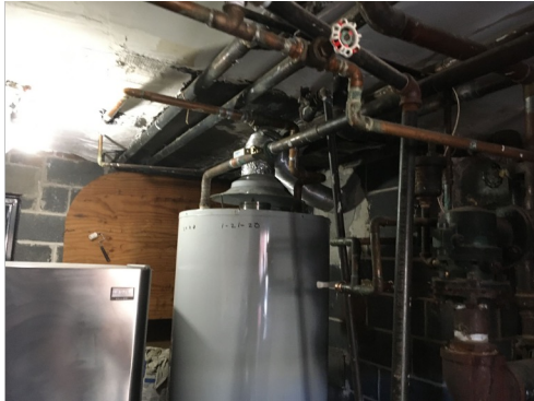
Existing Gas Water Heating
