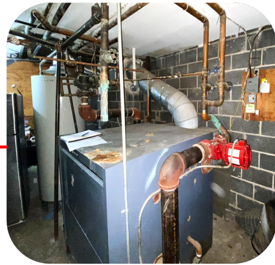
Existing boiler and gas HW heater
