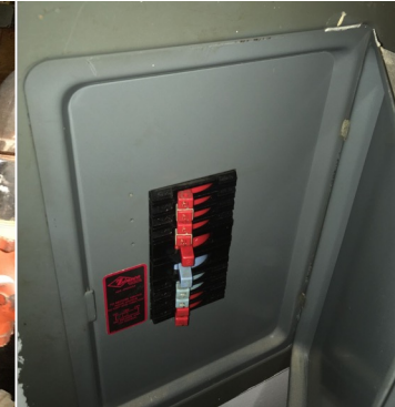
Existing 40 Amp Panel in Unit
