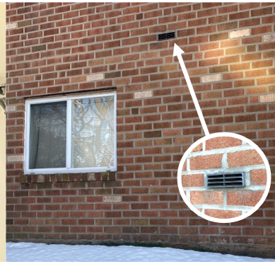
Existing Bath Ventilation
