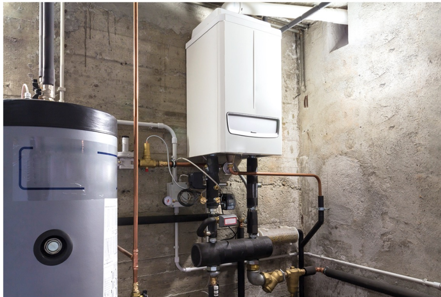
UK heat and hot-water systems examined contain an average of 9kgCO 2 e per kg of product weight
